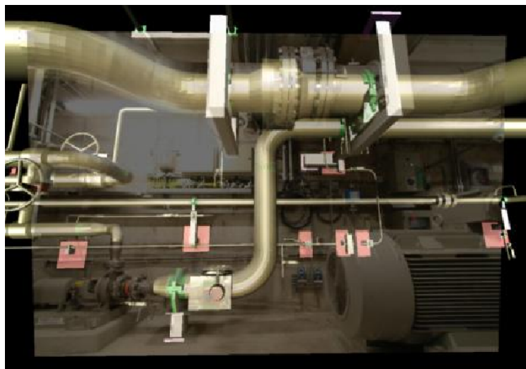
Figure 1.9.: Planning and change management. For referencing the indicated anchor plates are used. Their position is known with high accuracy. (Courtesy of Pierre Fite-Georgel [Geor 07])
